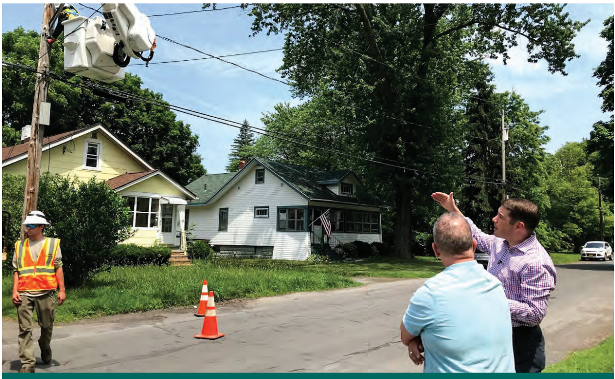
Mayor Ben Walsh discusses progress on city LED light installation process with contractors. Part of Mayor Walsh’s Syracuse Surge strategy, all light poles will have “Smart City” sensors, making them both energy efficient and cost effective, with Walsh estimating tax payer savings of approximately $3 million dollars. Photo Credit: City of Syracuse
