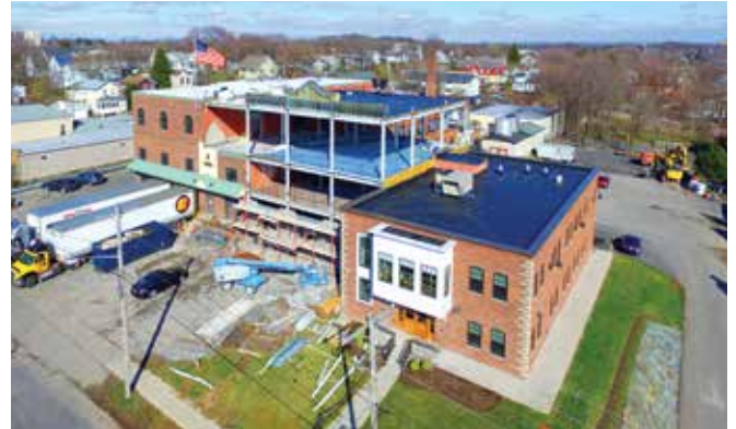
Cathedral Candle Company, on the north side of Syracuse, undergoes a $2.5 million expansion.
