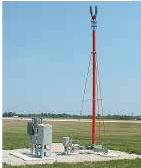
Saab Sensis remote units provide accurate and timely surveillance of aircraft flying around an airport and will be installed at select CenterState NY locations as part of the REDC funding, Round 4.
