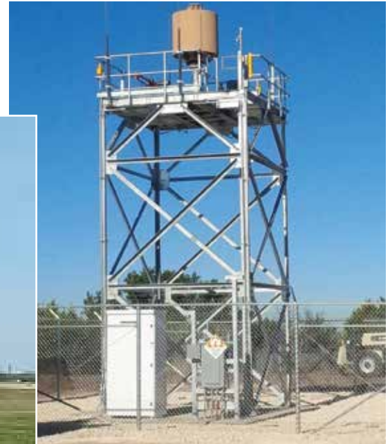
The first ground-based sense-and-avoid radar system is installed at Fort Hood, Texas, to support unmanned aerial systems operations out of Robert Gray Army Airfield. LSTAR (V)3 radars are part of the system that will be set up at Griffiss and other approved locations.
